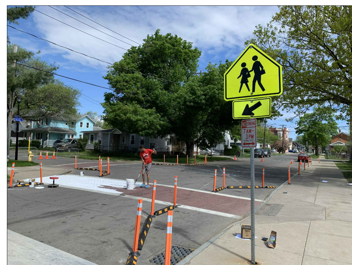
CURB BUMPOUTS AND DELINEATORS AT ORANGE AND ORCHARD
